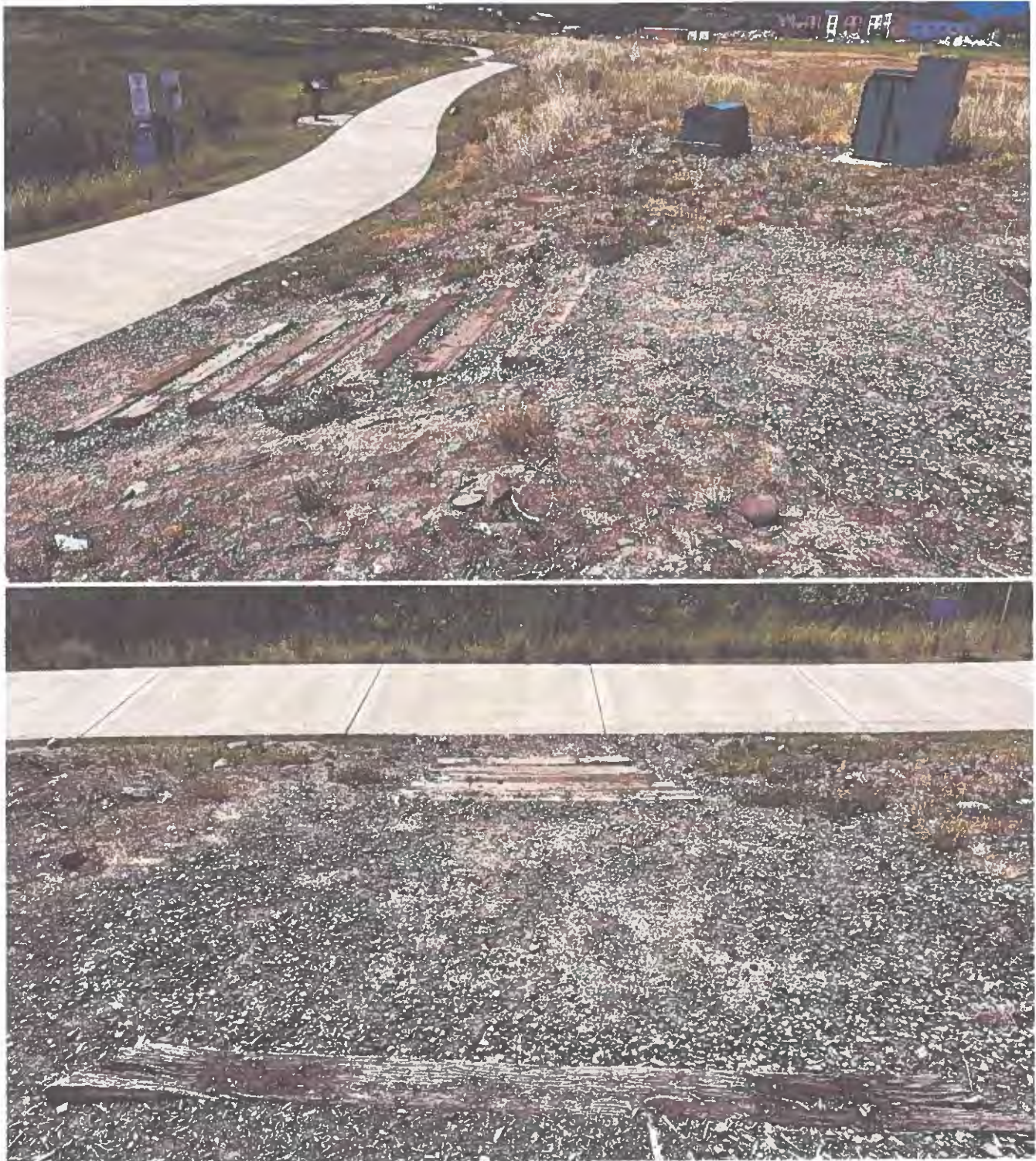
AARP Sponsorship – Senior Center Riverwalk Staircase & Handrail – Before
