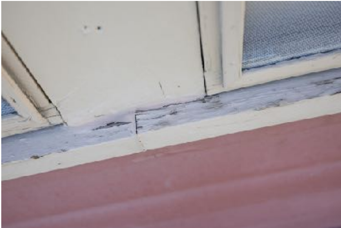
East side showing rotted wood and peeling paint
