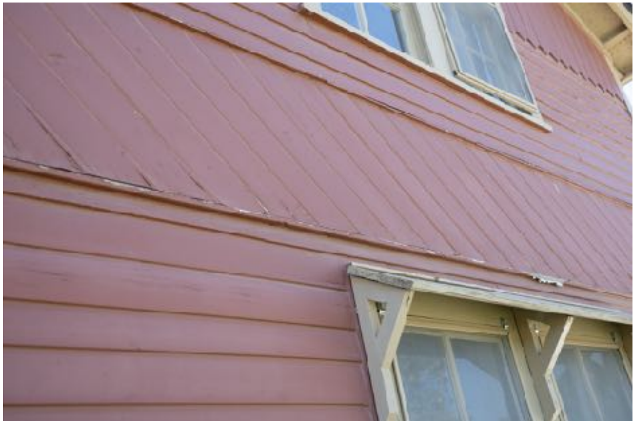
East side showing rotted wood and peeling paint on upper level
