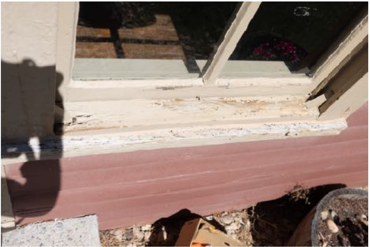
West side window trim damage and peeling paint
