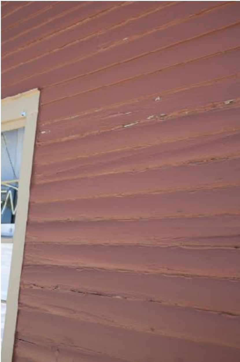
North side peeling paint
