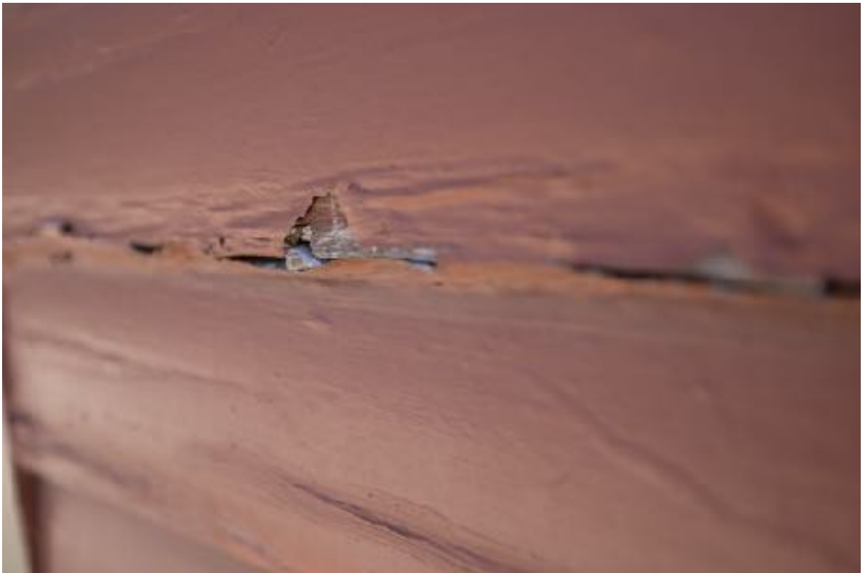
North side damaged siding and peeling paint
